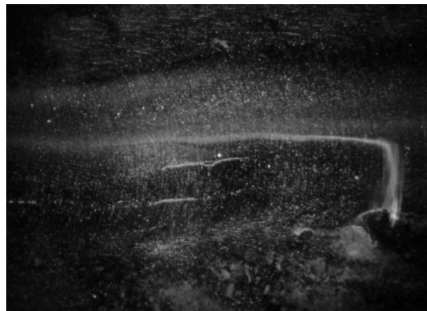
Fig.7. Visible detected crack with the length of 10mm on the line of the fusion butt joint at the weld in the area ["X"].
