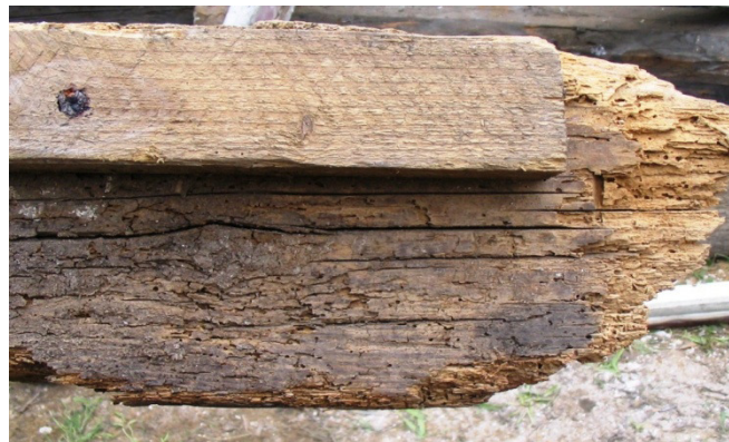
Fig. 1. Damaged ceiling beam end. Wood decomposition due to fungi.
