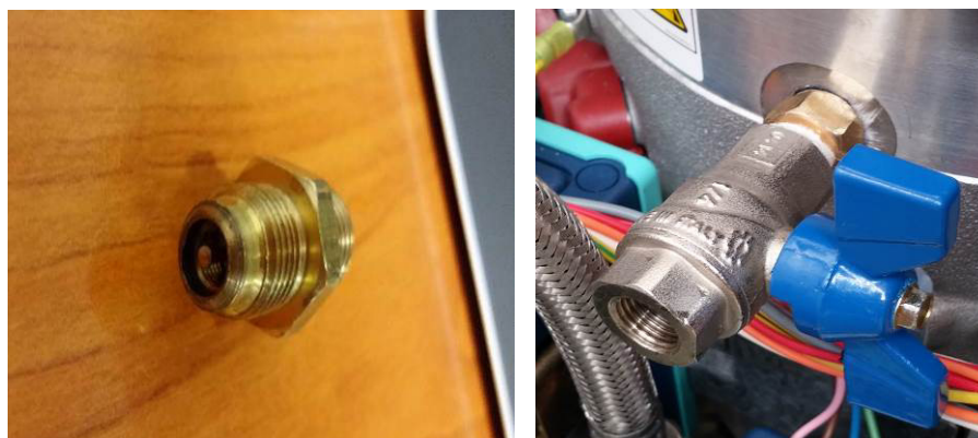
Fig. 5 Defective supply working gas valve and new system of working gas supply
