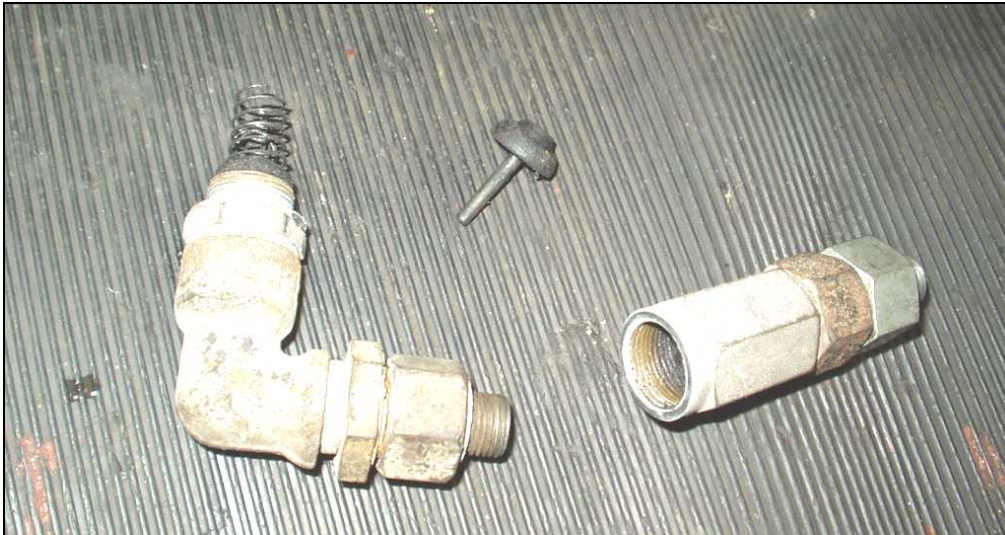
Fig. 4. Dismounted return valve with damaged gusset and sealing rubber band.
