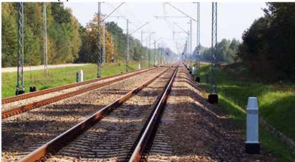
Fig. 1. Views fragment main railway E-20 Minsk Mazowiecki-Siedlce with installed preventers UOZ-1 [2, 7]
