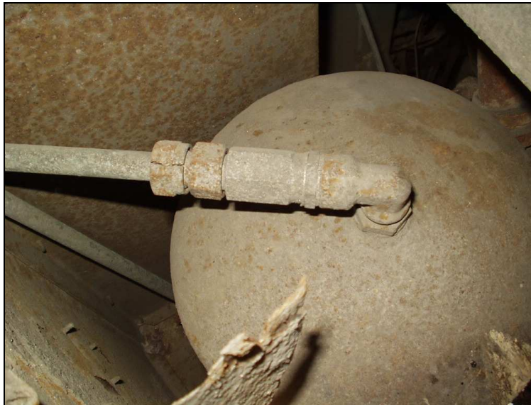
Fig. 3. Return valve still installed at the air receiver of the bus.
