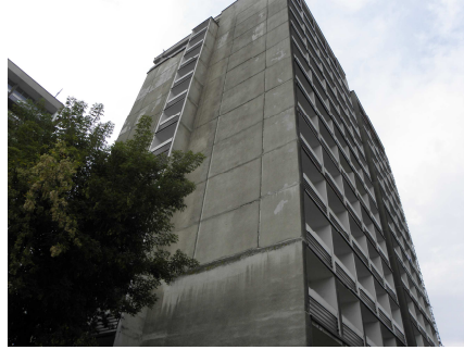
Fig. 2. End wall of students' house no. 2 of the Physical Education University in Cracow.
