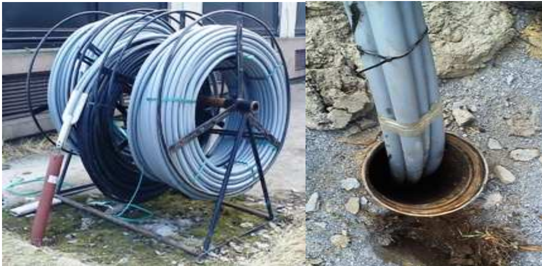
Fig. 1. Vertical earth heat exchanger with a probe and a load introduced into the borehole
