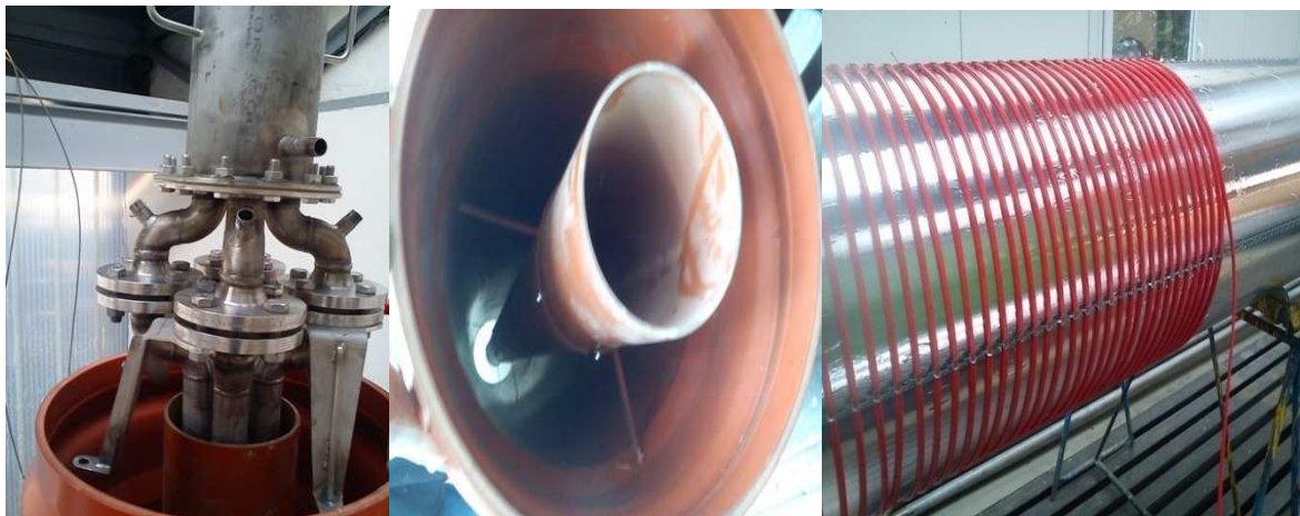
Fig. 3. Installing a heat exchanger system to "pipe in pipe" heated by electric cables
