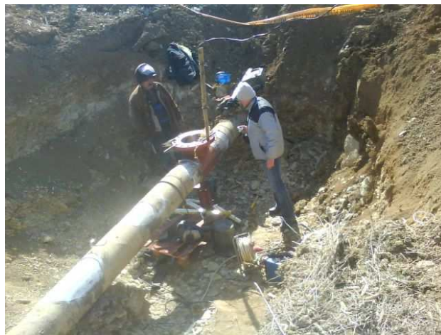
Fig. 2. Remote on the place, where fitting was installed on gas pipe in cutting.
