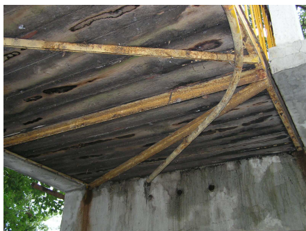
Fig.1 Bridge floor corrosion
